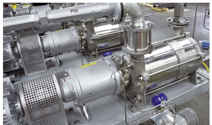
VHCM (ChemTAL) liquid ring vacuum pump as per TA Luft with a pump monitoring system used for solvent recovery.
